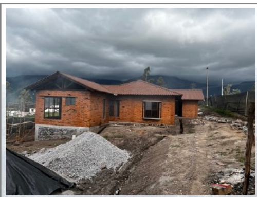
Roof is on and windows have been installed. Now just awaiting the doors and some other finishing touches.
